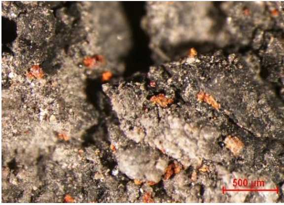
Fig. 16 – B2-(0-5mm), Development of the cracked surface with partial oxidation of the fine aggregate
