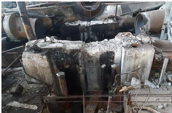
Fig. 2 – Spalling and crushing of top chemical grout along with underneath concrete and black stains of the fire-damaged face of Pedestal B2
