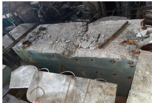
Fig.3 – Spalling and crushing of top chemical grout of Pedestal B4
